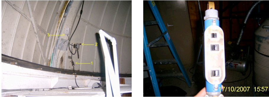
Figure 11: Left: The power supply cable and the switches that open the upper and lower shutters at the 84cm telescope. Right: The hand paddle that moves the telescope and the dome.
