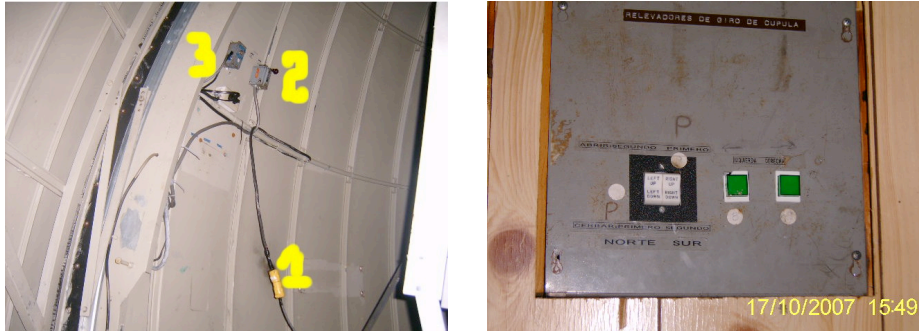
Figure 12: Left: The power cable and the switches that open the upper and lower shutters at the 1.5m telescope. Right: The switches that open the primary mirror shutters and that move the dome.
